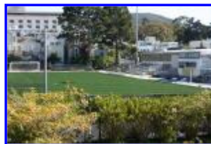
Negoesco Stadium ProTurf Project, 2010 - New turf laid in place and ready to be sewn together.
