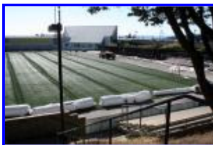
Negoesco Stadium ProTurf Project, 2010 - New turf laid in place and ready to be sewn together.
