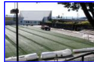
Negoesco Stadium ProTurf Project, 2010 - New turf laid in place and ready to be sewn together. Additional new turf rolls ready for installation on sidelines.
