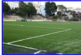
Negoesco Stadium ProTurf Project, 2010 - New turf laid in place, lines complete. Tractor at midfield spreading rubber pellets.
