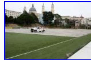
Negoesco Stadium ProTurf Project, 2010 - Old turf removed from half of the field.
