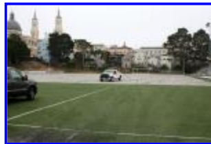
Negoesco Stadium ProTurf Project, 2010 - Old turf removed from half of the field.
