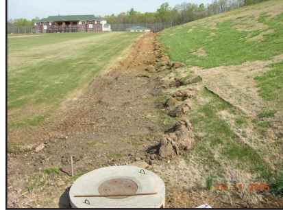
Example of bad conduit installation along edge of a natural turfgrass field and reconstruction to fix it. Photo: Tony L. Strickland, CSFM
